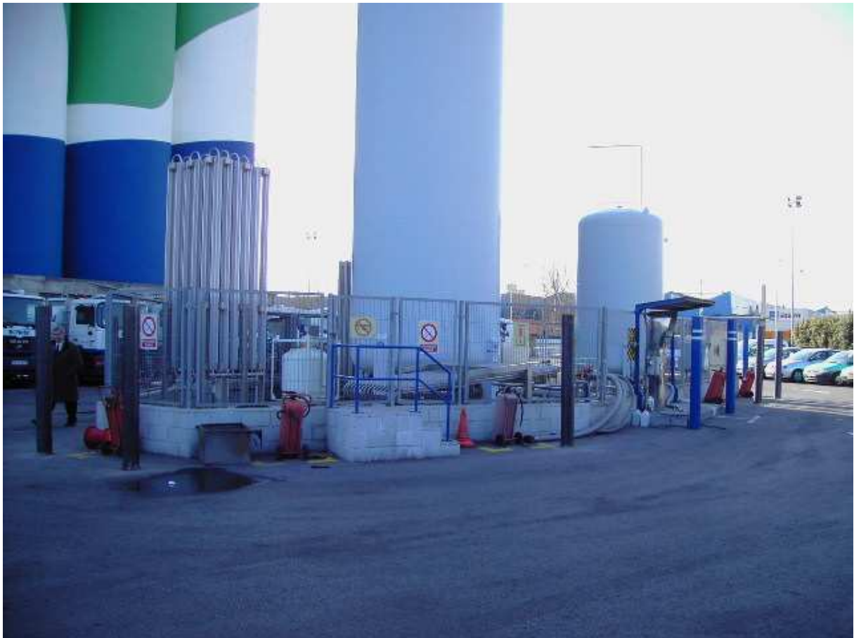
Fig.1 Privat LNG refuelingstation in Barcelona Spain for 35 refuse trucks as an example.
